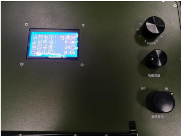
1. Current Voltage: Power Off Status
